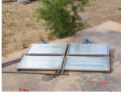
Figure 2. Winston Series CPC Solargenix® Collector
