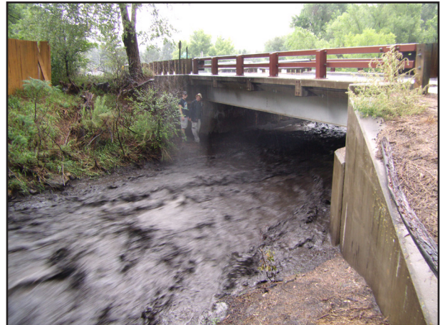
Figure 26. Fires increasing flooding.
