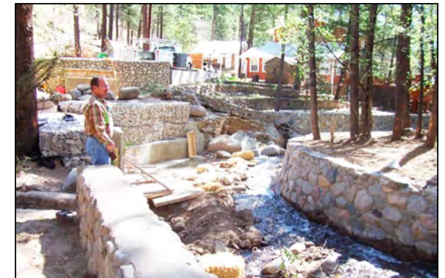
Figure 3. Following multiple attempts at bank stabilization to protect encroaching urban infrastructure, the Rio Ruidoso has been reduced to a concrete canal with loss of all natural function except water transport.
