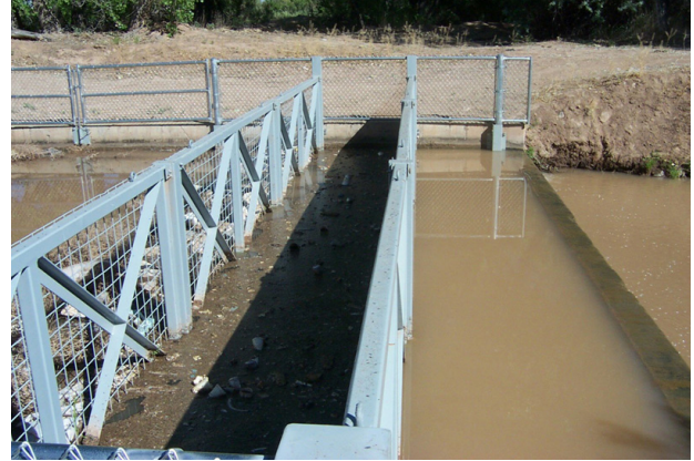
Figure 13. La Orilla Outlet Debris Baffle
