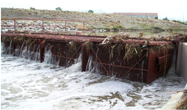
Figure 15. Bear Canyon Arroyo Debris Screen
