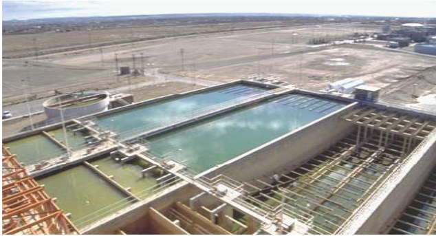
Figure 6. Rapid Mix Flocculation, Settling: Ferric chloride coagulation destabilizes turbidity and disinfection byproduct precursors, providing 95% turbidity removal and up to 50% disinfection byproduct precursor removal.
