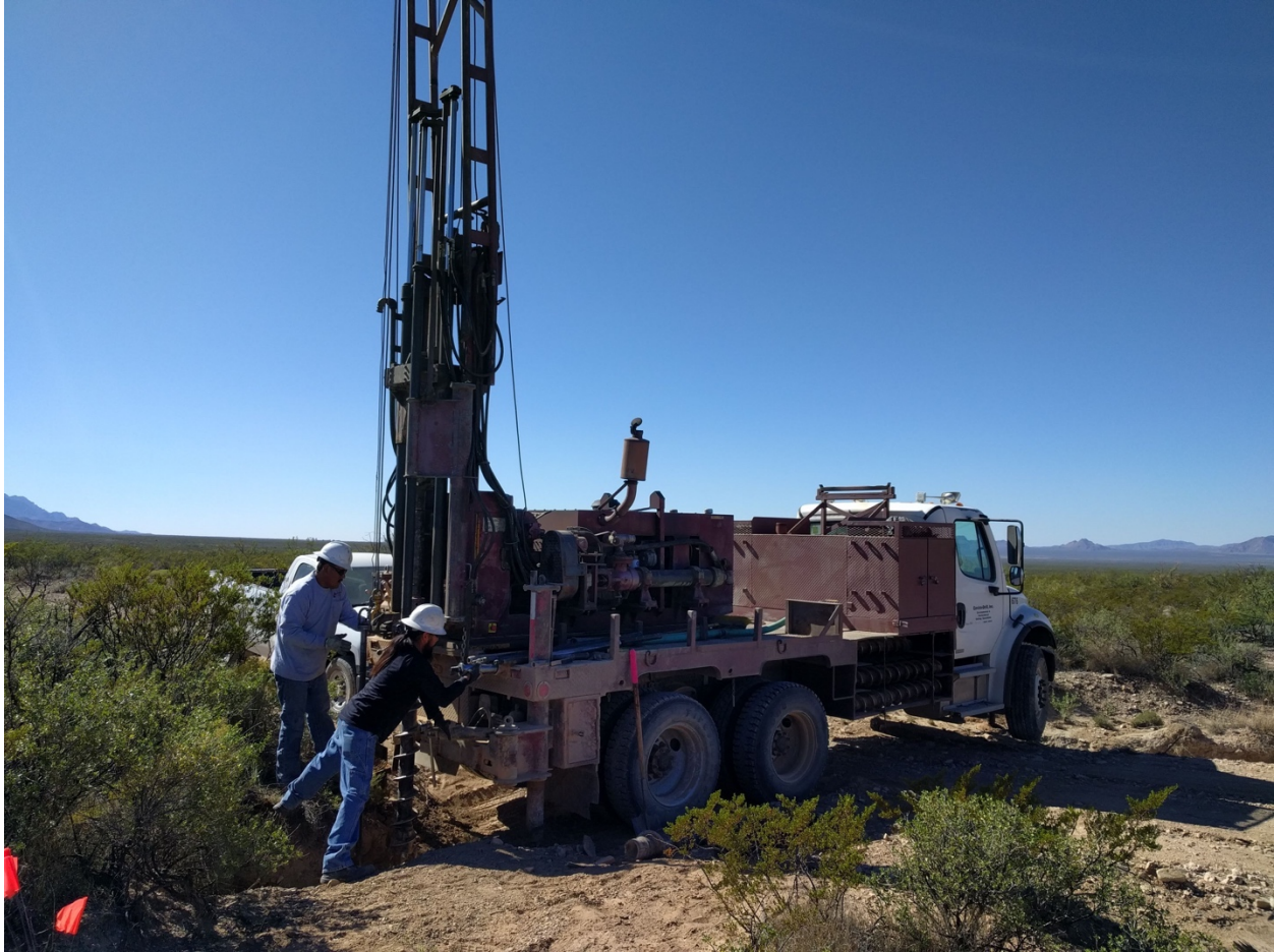
Figure 8. Drill rig activity at core site Channel-A. The road slightly dams the channel at this location, meaning the core is being extracted from a local depression that collects water during runoff.
