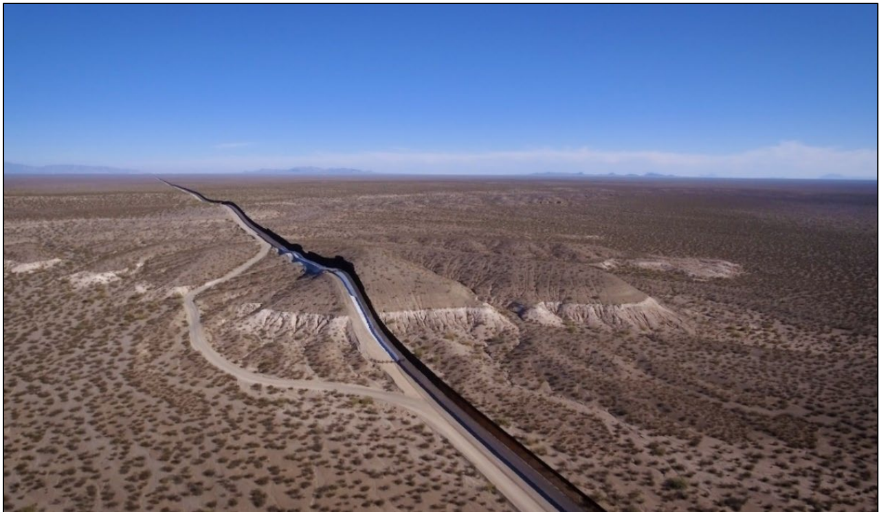
Figure 1-14. (courtesy of PBS-New Mexico in Focus—Our Land) Fall 2019 aerial photograph of a newly completed section of the US-Mexico Border Wall in the southern Mesilla basin at the 31° 47' N Parallel ( cf. Fig. 1-15 ). El Paso del Norte is on the eastern horizon between the Franklin Mountains and Sierra Juárez Uplifts. The photo site near the 107° W Meridian depicts a typical Chihuahuan Desert landscape in southern Doña Ana County, and northern Municipio de Juárez.
