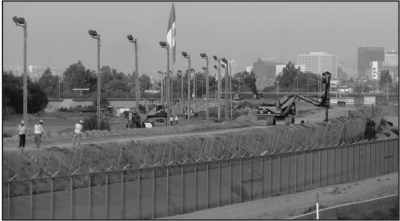
Figure 15. Example of construction of the border fence with workers in El Paso between the U.S. and Mexico, 2009.
