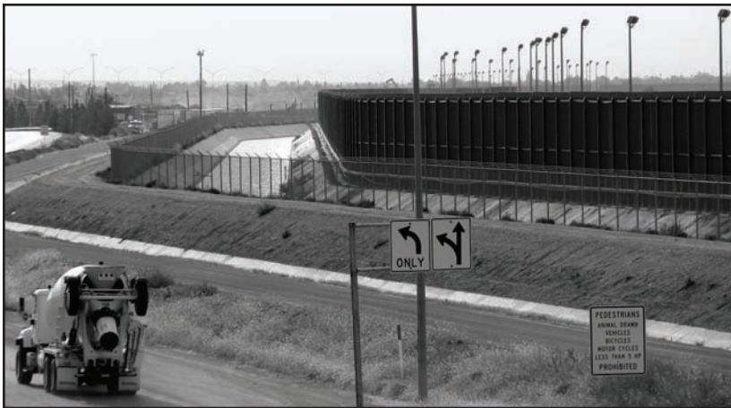
Figure 14. Example of construction of the border fence in El Paso between the U.S. and Mexico, 2009.
