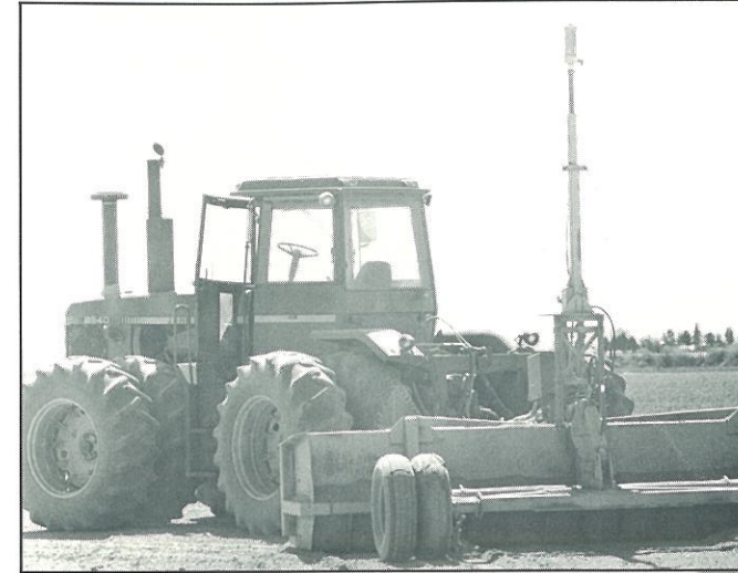
The laser-leveling technique uses a rotating laser beam mounted on a command post that transmits signals to a receiver mounted on the tractor's scraper, directly above the cutting blade. The laser beam controls the scraper's action and can be set to any desired grade. (Photo by New Mexico Water Resources Research Institute)
