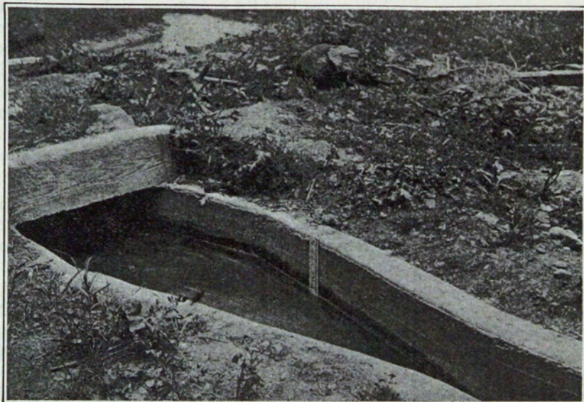
Figure 20.—One-foot reinforced concrete Parshall measuring flume set in close proximity to farm lateral headgate. Free-flow discharge of 2.53 second-feet. Lake Canal, near Fort Collins, Colo.
