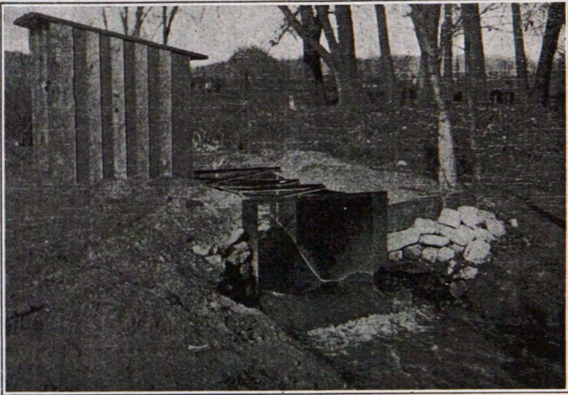
Figure 27.—Three-foot metal Parshall measuring flume discharging about 5\frac{1}{2} second-feet. Sewer outlet, city of Colorado Springs, Colo.
