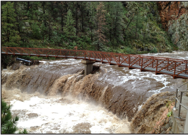
Figure 20. September 2013 flooding of Gallinas Creek.
