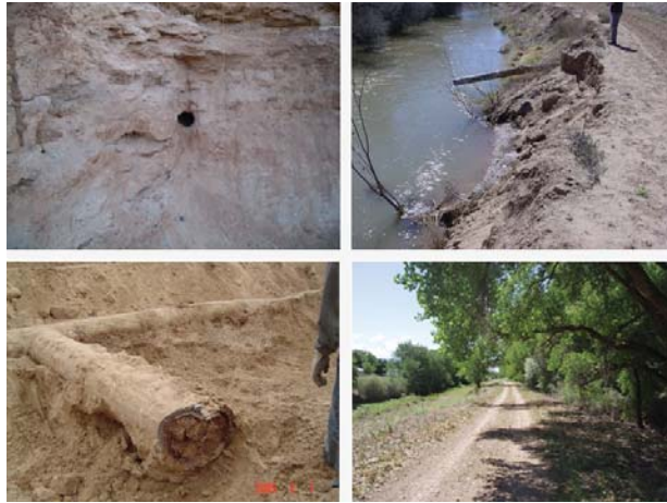
Figure 3. Current Albuquerque levee conditions
