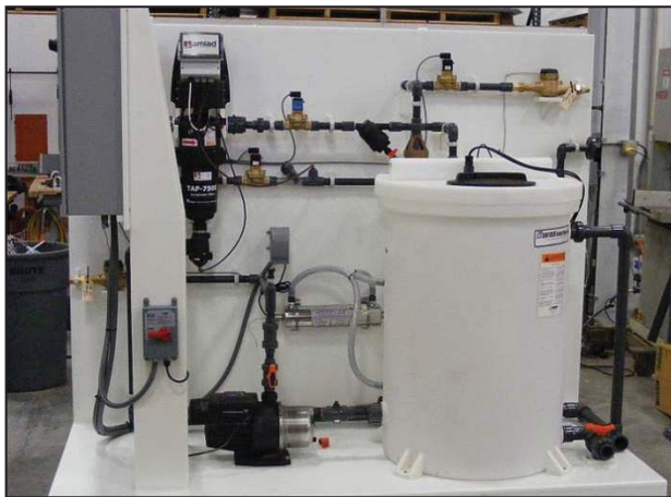
Figure 16. New active mechanical rainwater harvesting
