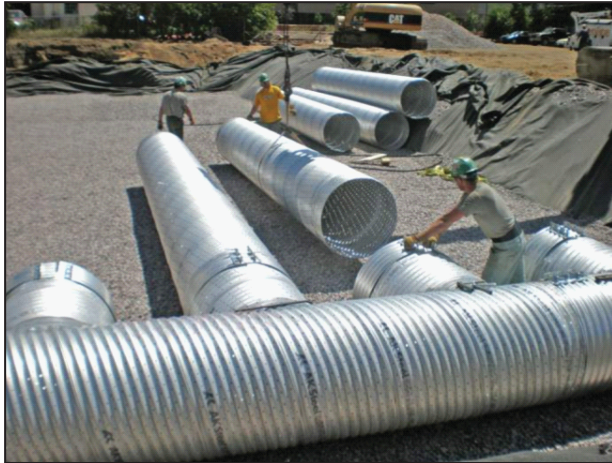
Figure 19. Impermeable pond liner in the background and perforated metal pipe that will be filled with gravel and wrapped over the top, similar to the chamber system
