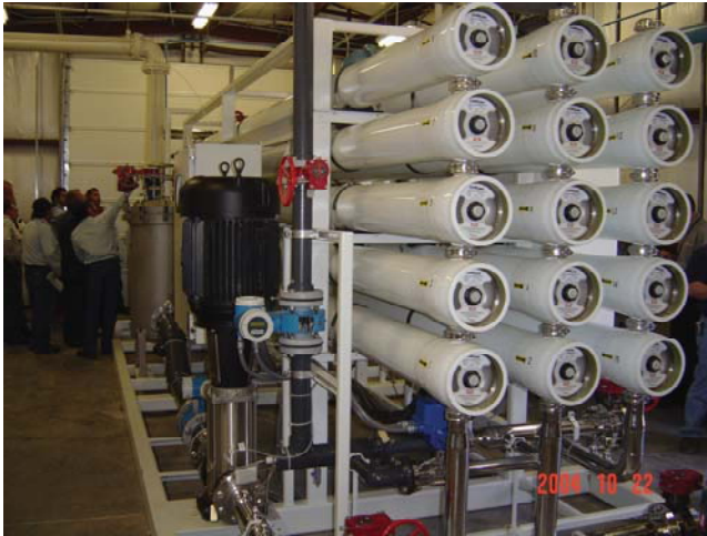
Figure 9. Reverse osmosis desalination unit in El Paso
