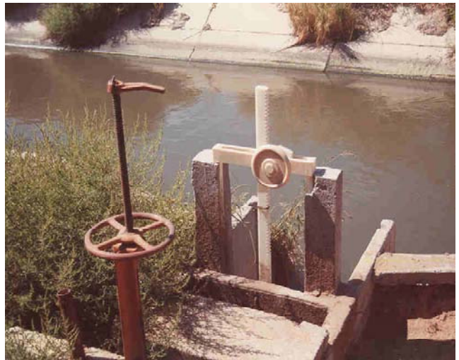
Figure 8. Irrigation head gate damage by salt
