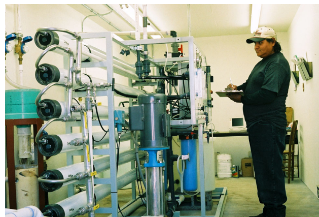
Figure 5. White Cliffs RO Plant
