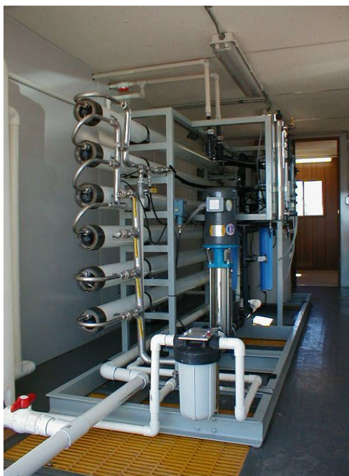
Figure 3. Typical Small RO “SKID”
