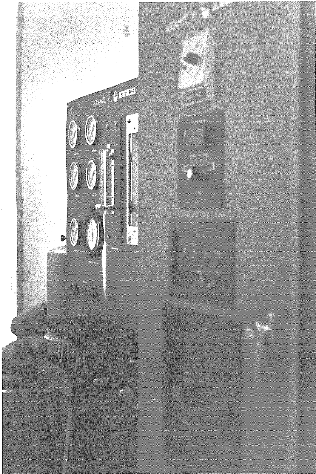
Figure 19. Electrodialysis Control Panel
